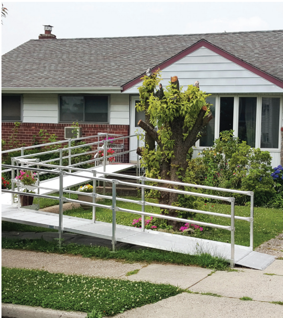
Handicapped ramp that was installed through the Town's Community Development Block Grant Program.
