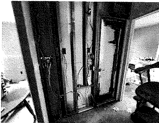
Interior (First Floor) – Unfinished wall, exposed wiring and incomplete electrical work. Debris and trash on floor.
