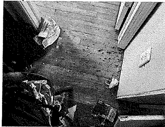
Interior (First Floor) – Evidence of vermin infestation.
