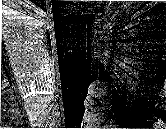
Entry (First Floor) – Personal items and trash in floor. Flooring damaged and dilapidated, in need of maintenance.
