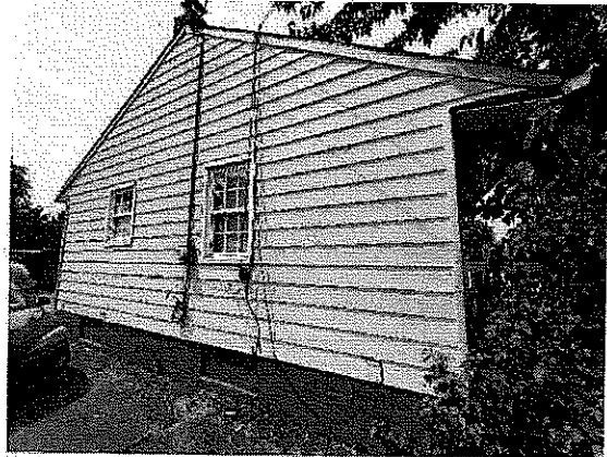
Side Façade (East) – Exposed / dangling wiring. Rusted electric meter. Foundation cracks.
