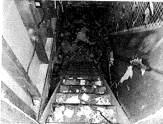
Interior (Basement Stairway) – Household items, trash, and debris on floor and stairs. Unsanitary / uninhabitable conditions.
