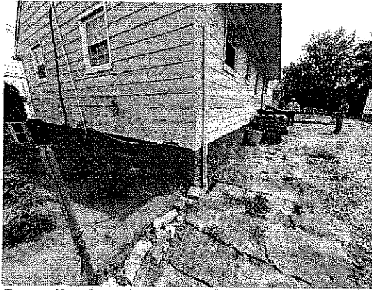
Corner (Southwest) – Exposed / dangling wiring. Missing soffit. Foundation cracked. Fascia dilapidated. Holes in siding, damaged siding. Hanging PVC pipe.
