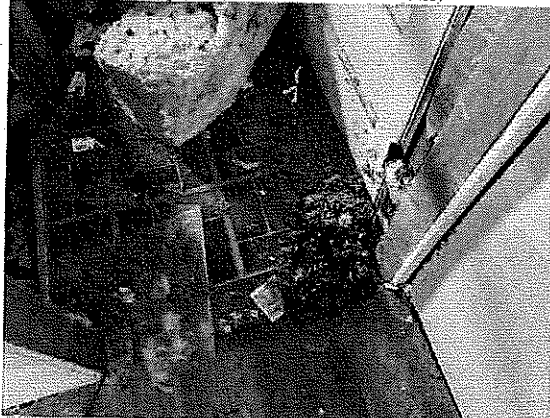
Interior (First Floor) – Evidence of vermin infestation. Building supplies and debris on floor. Unsanitary / uninhabitable conditions.
