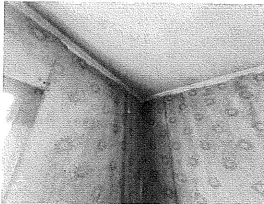
Interior (First Floor) – Evidence of water damage behind wallpaper. Wallpaper peeling away.
